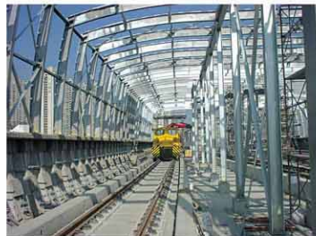
West Rail High Tension Cable Guard & Noise Enclosure 西鐵高壓電纜保護及隔音屏障
